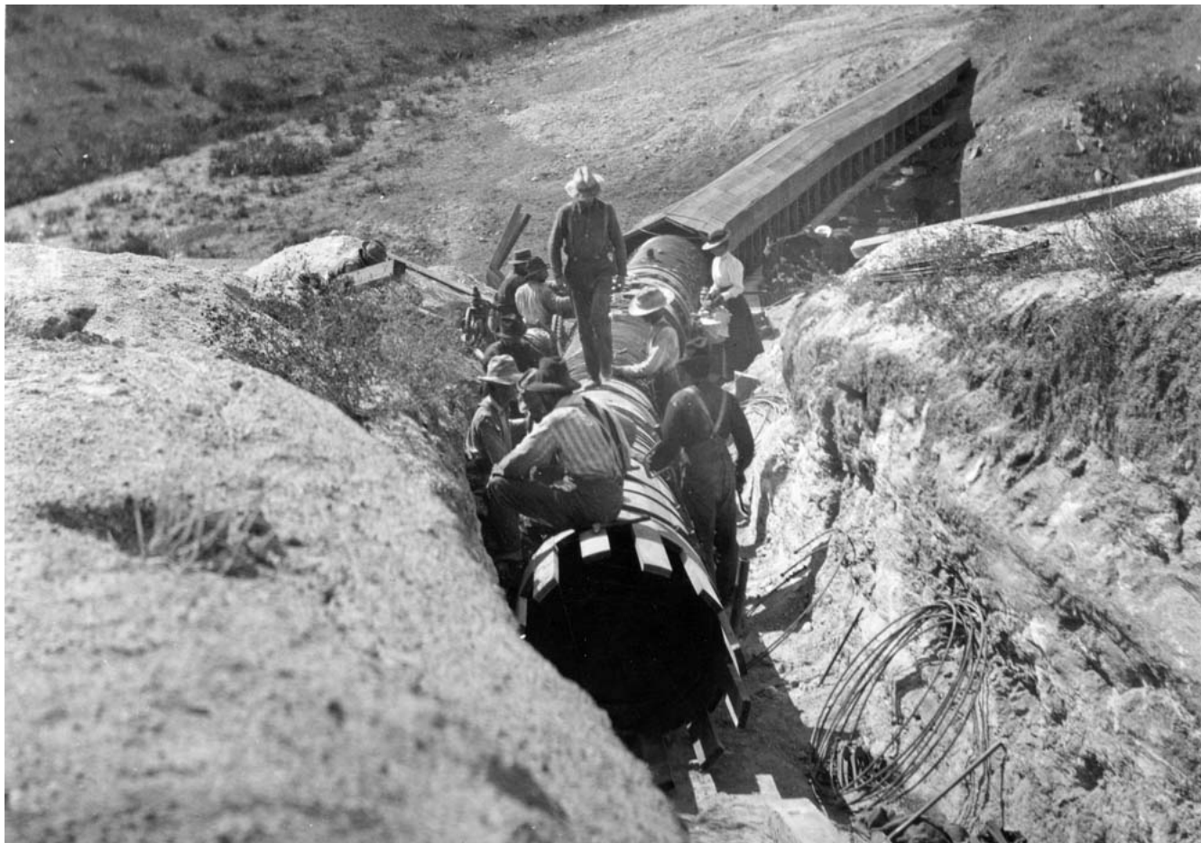
SCMW workers laying 40-inch wood water pipe from the Lower Otay ca. 1901 ( Mary C. Oswell collection, Bonita Museum )
