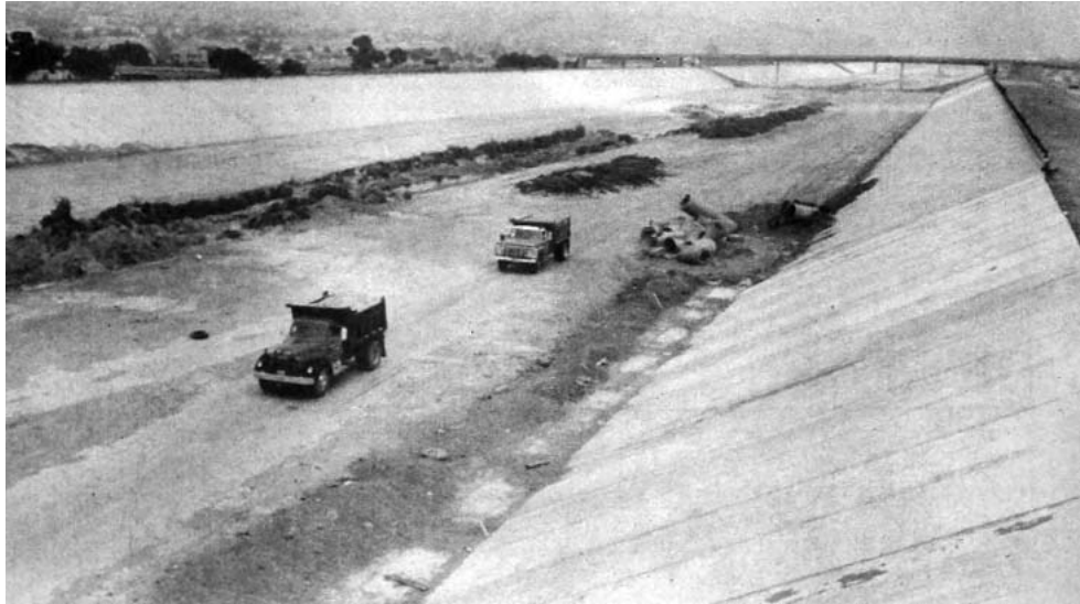
Tijuana flood control channel under construction on Mexican side. (Chula Vista Star-News, July 22, 1976)
