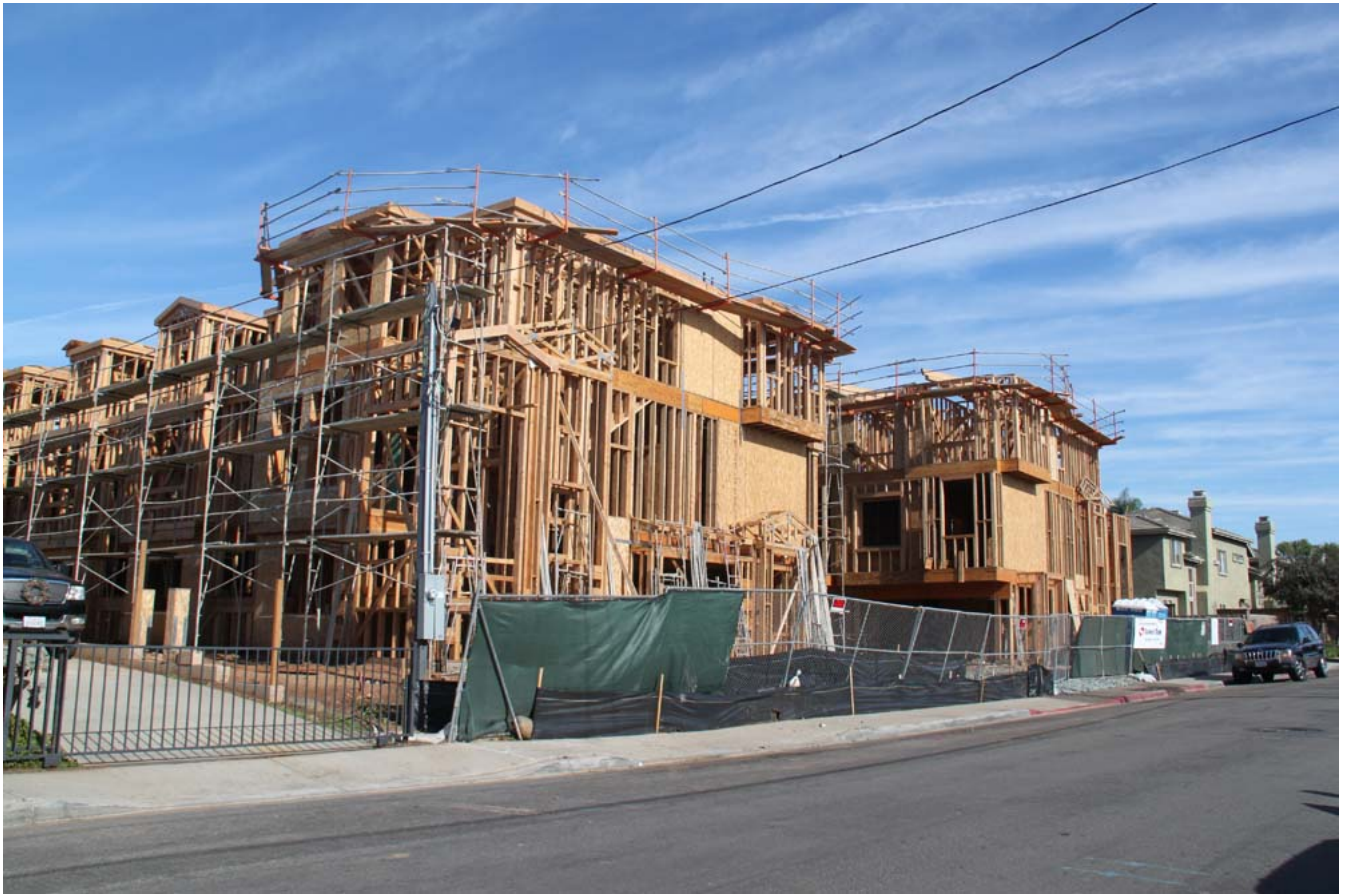
The potential historic house at 778 Ada Street has been demolished for the construction of the Ada Villas townhomes.
