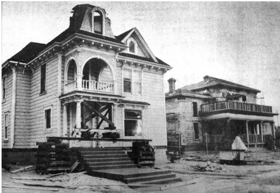
The Kimball house and the Elizur Steele house under renovation after being moved to Heritage Square
